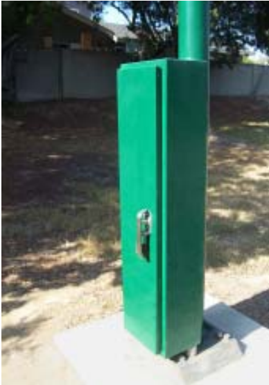
SECURE NEMA 12 CABINET
