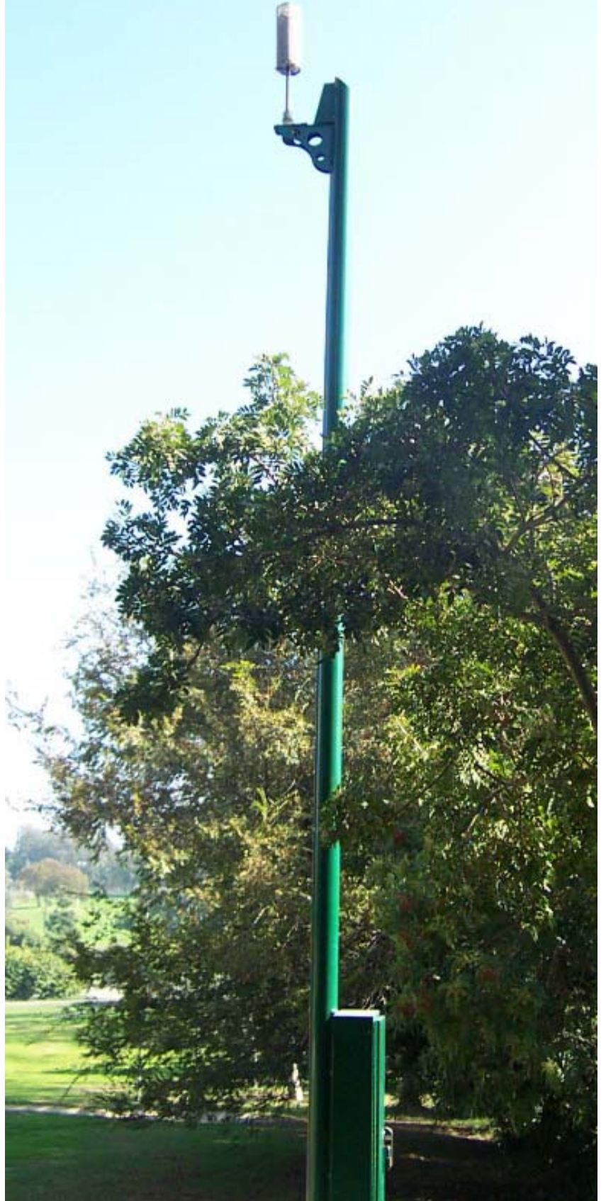
SYSTEM SHOWING CABINET & MICROPHONE POLE
